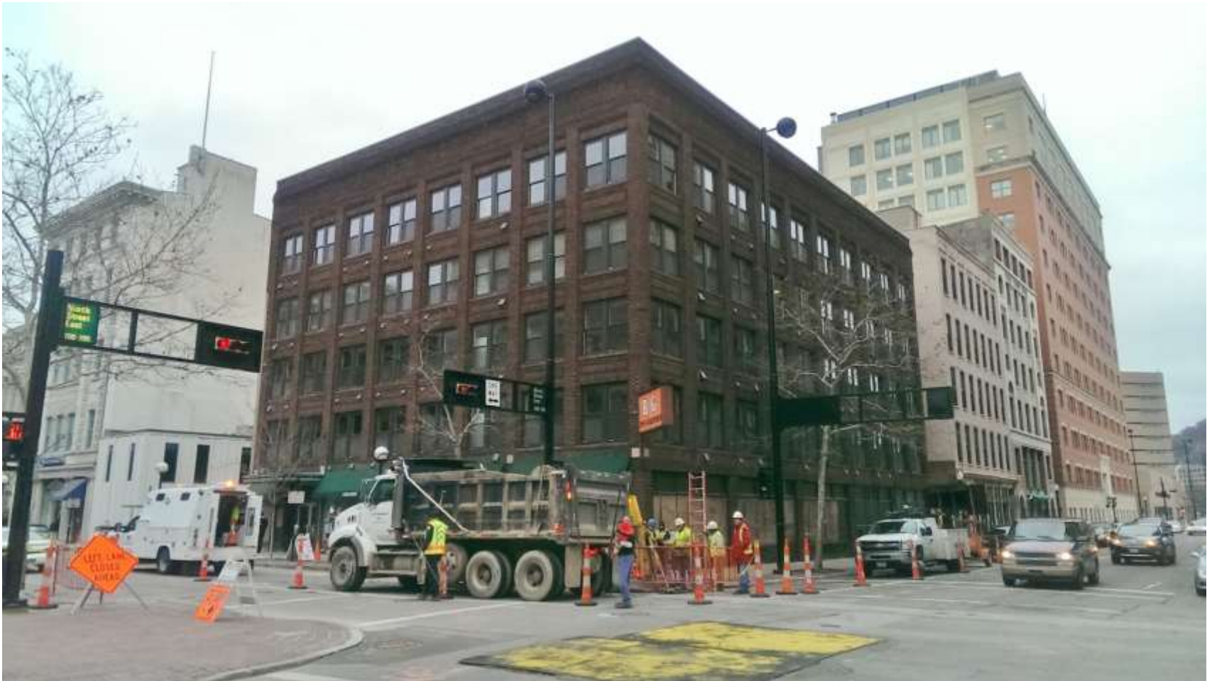
Watermain tie-in at 9th & Main adjacent to office building just converted to apartments
