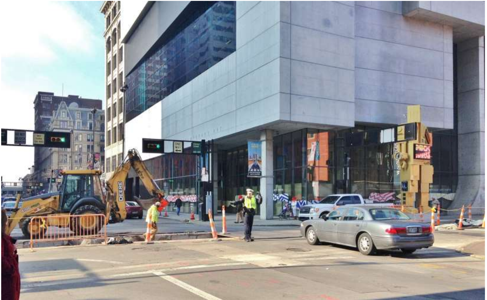
Cincinnati Police assist traffic movement during Walnut Street track slab work at 6th St.
