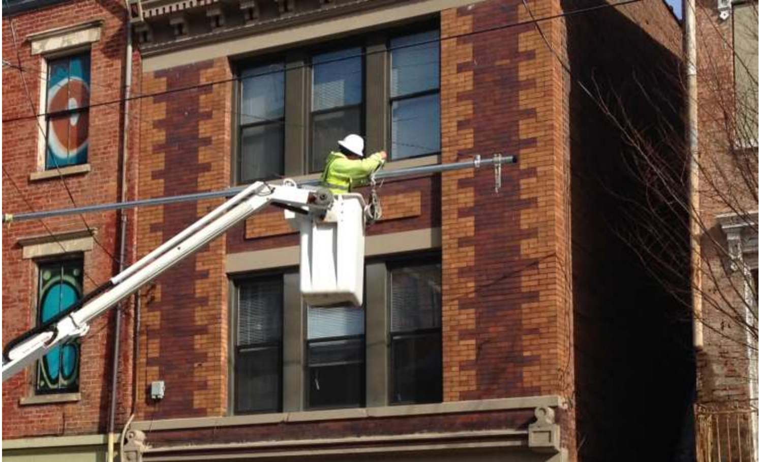
Rigging an OCS bracket prior to contact wire pull on Elm Street
