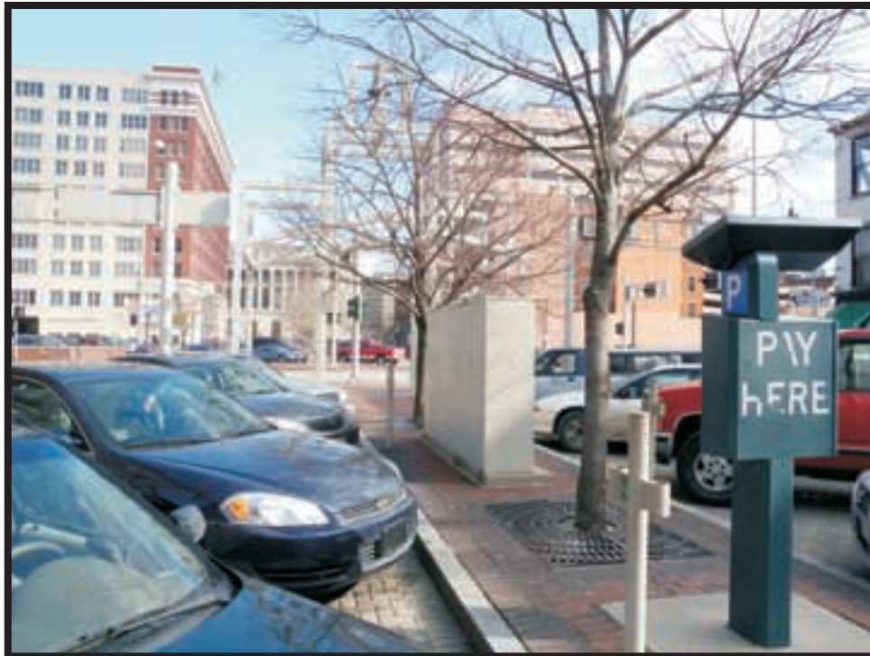
Plate A53. View of Proposed Substation Location west of Walnut Street on Court Street.
