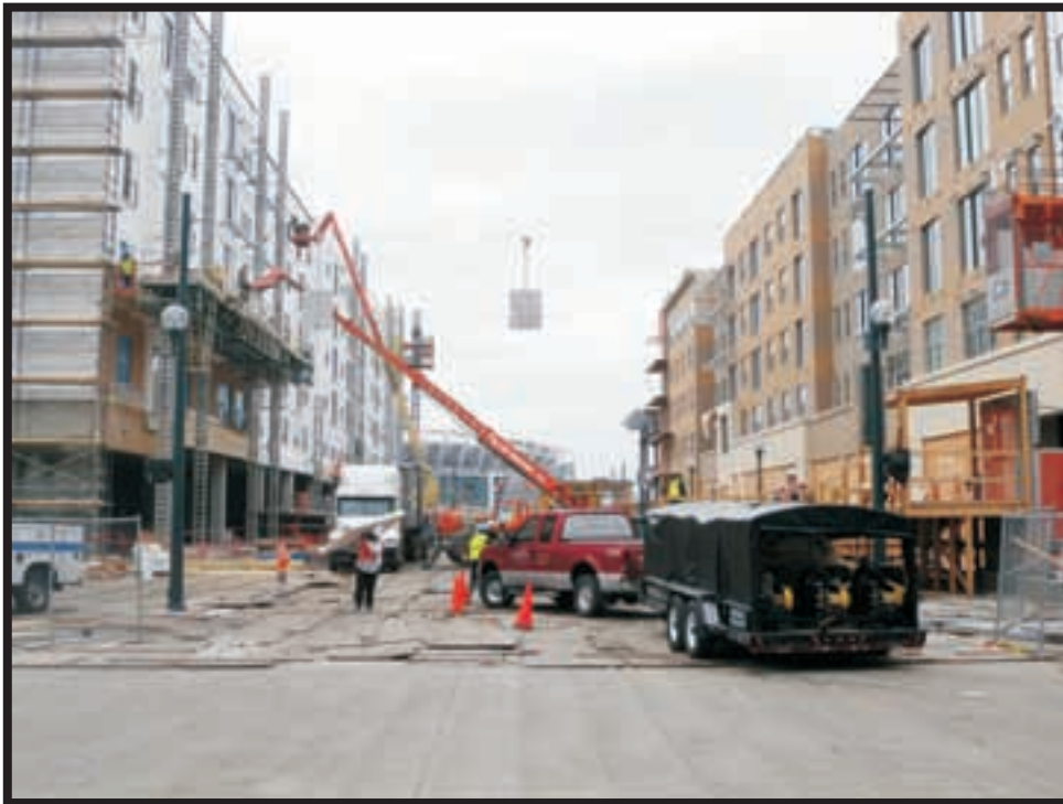
Plate A30. View of Proposed Streetcar Stop Location 1 at East Freedom Way, facing west. Note construction prohibited a photograph of the exact location.
