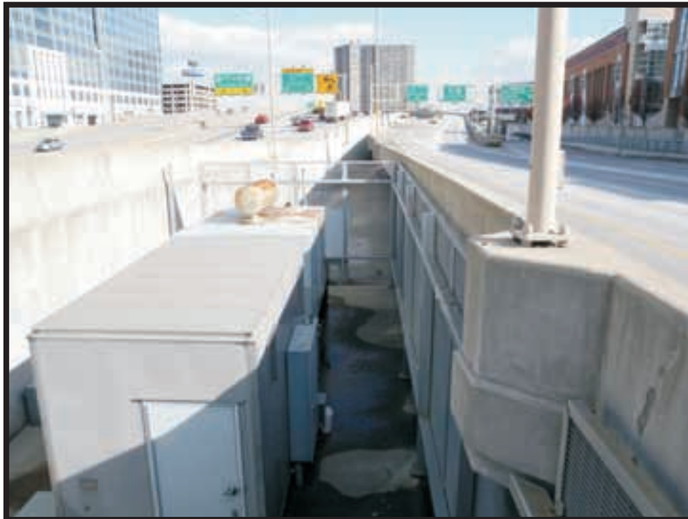
Plate A52. View of Proposed Substation Location between Second Street and eastbound Fort Washington Way (I-71) just east of Main Street.
