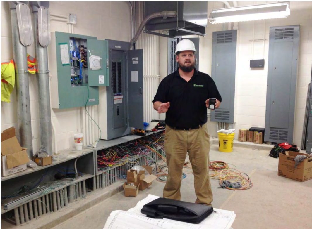
Photo 11: Training on the MOF lighting control system
