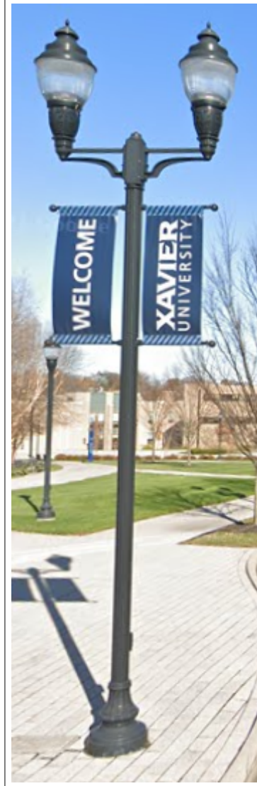
Decorative pole lights
