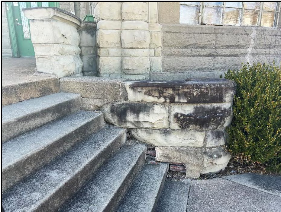
Figure 4. Walls and steps to be removed at location of ADA ramp connection. Photo by Staff.
