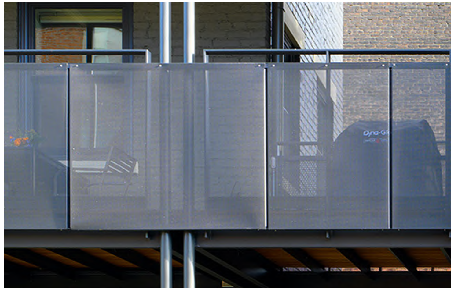
PERFORATED STEEL GUARD WITH STEEL STRUCTURE BEHIND Artichoke OTR 1824 Elm Street
