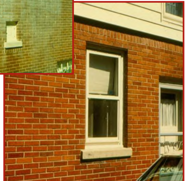
AFTER CLEANING WITH 101
