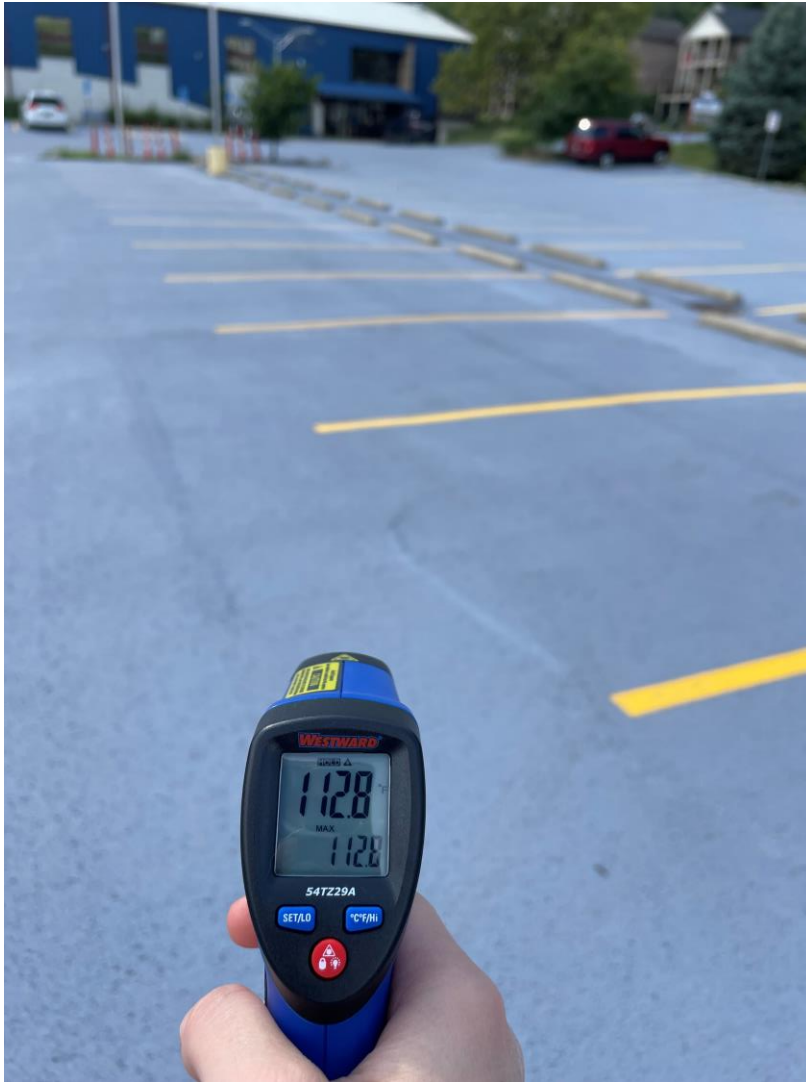
Surface temperature of the parking lot with CoolSeal at LeBlond Recreation Center on 8/25/23 when ambient temperature was 95 F.
