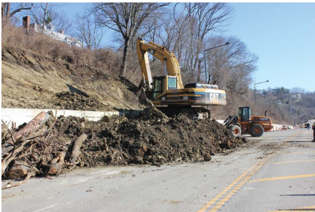
Severe storms in 2016 resulted in landslides on Columbia Parkway. Hillsides are one type of sensitive land-use areas in Cincinnati. Photo courtesy of City of Cincinnati.
