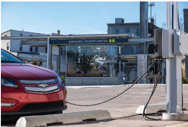
The Northside Transit Center features electric vehicle chargers that are available to the public. Photo courtesy of Metro.
