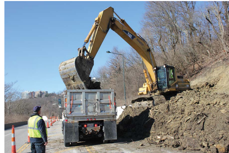
Intense storms caused landslides onto Columbia Parkway in 2016, requiring over $17 million to clean-up and repair. Photo courtesy of City Staff.
