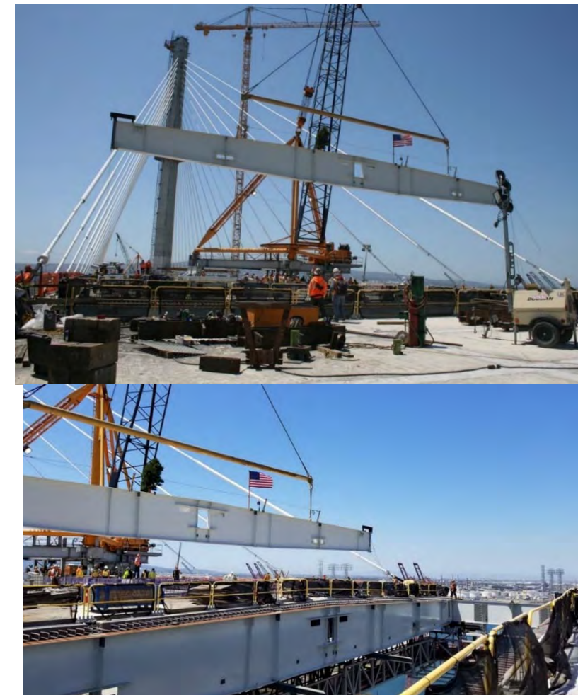
Figure 8: Installation of floor beam for the New Gerald Desmond Bridge in California using an erection crane.
