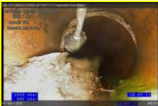
[Grade 2] Deposits Attached Other at 009.6 ft, 7 - 9 o'clock | Mud in line
