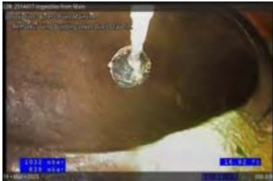
Access Point Mainline at 000.0 ft | Tving building sewer due to cave in.
