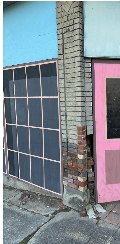
BRICK CONDITION - NORTH EAST CORNER
