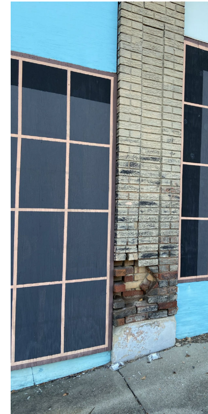
BRICK CONDITION - AUBURN AVENUE PILASTER
