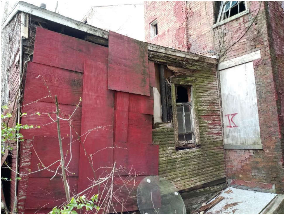
Figure 7 South facing side of rear addition where it meets the brick structure
