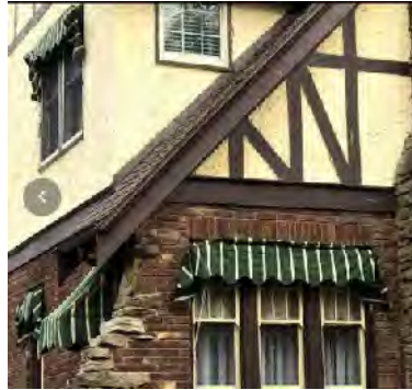
Accurate canopy location, installation and material
