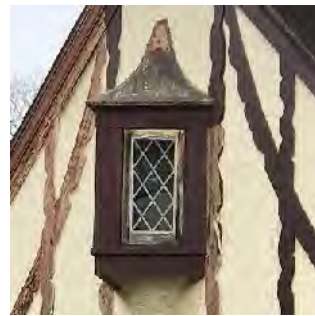
Wood window in poor condition
