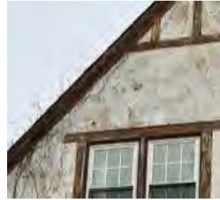
Masonry in poor condition
