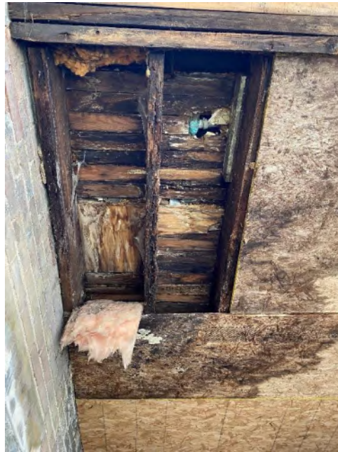
Photo 16 – Damaged Bathroom Floor Framing from Covered Entryway
