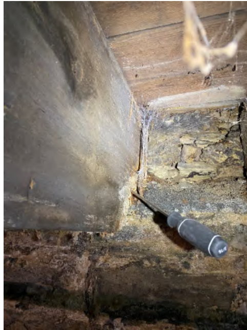
Photo 6 – Soft Rotted Joist Bearing End, Left Foundation Wall
