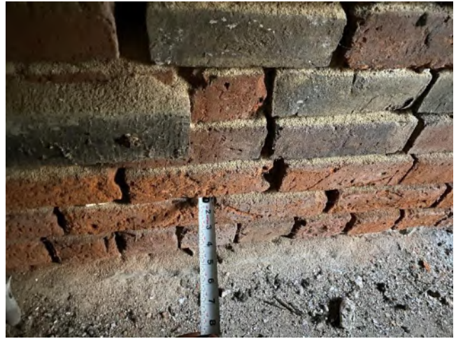
Photo 6 – Eroded Basement Wall Joint Depth Measurement
