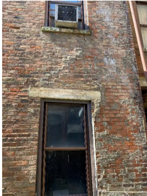
Photo 18 – Rear Exterior Settlement Cracking Above Settled Foundation Corner
