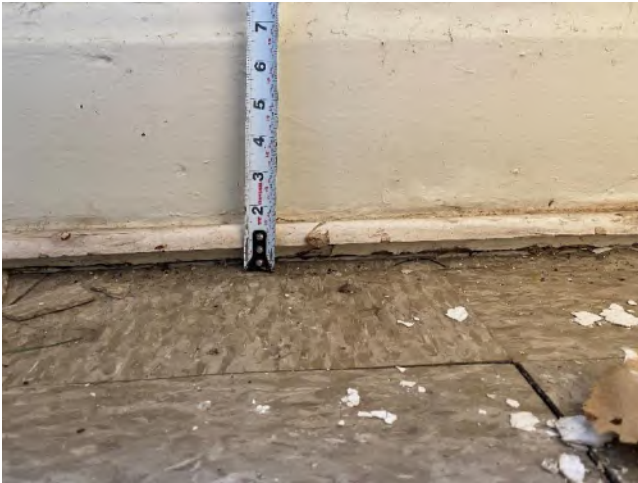
Photo 17 – Evidence of Floor Drop at Damaged Bathroom Floor Joists
