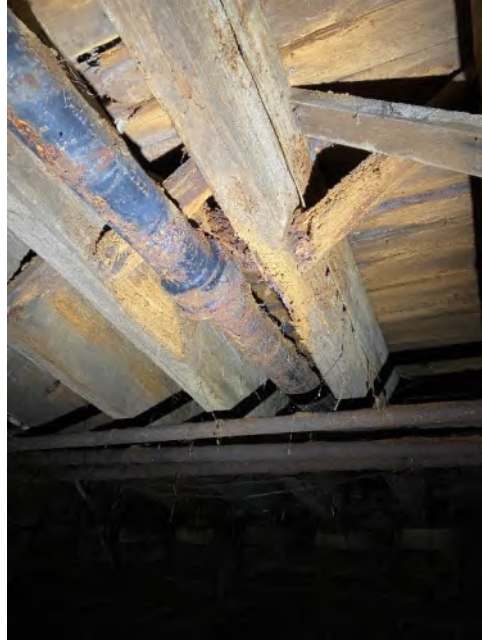
Photo 10 – Moisture Damaged First-Floor Joists, Rear Basement Area Near Plumbing
