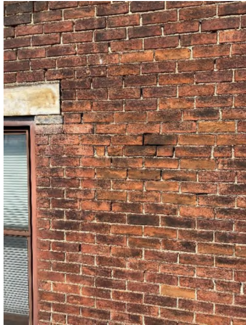
Photo 26 – Brick Joint Weathering, Upper Left Exterior
