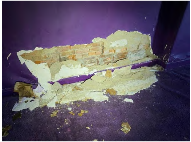
Photo 14 – Spalling Plaster, First Floor Level, Center Wall
