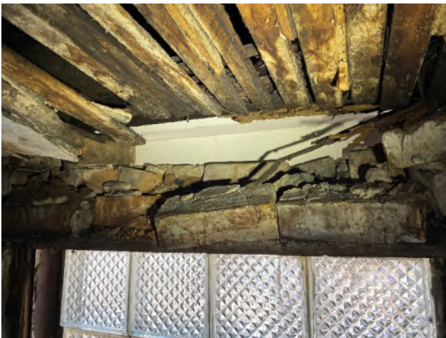
Photo 27 – Previous Water Damage and Missing Header, Front Attic Window
