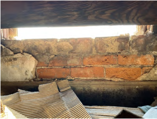
Photo 25 – Weather and Interior Brick Sill from Missing Window, Attic Level
