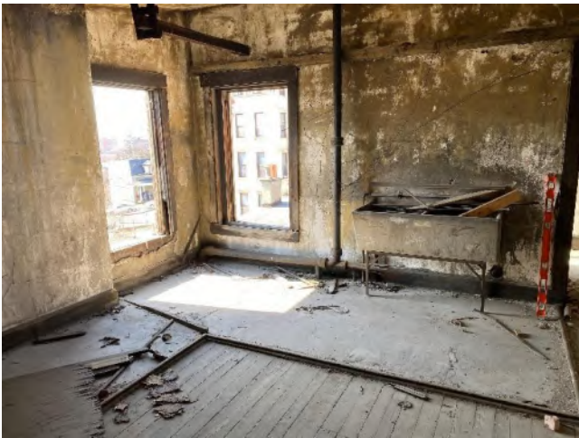
Photo 15 – Left Attic Space, Missing Windows
