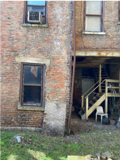
Photo 11 – Settled Rear Foundation Corner at Downspout
