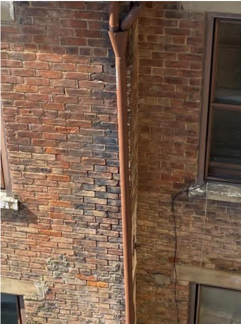
Photo 21 – Brick Joint Erosion at Downspout, Rear Exterior
