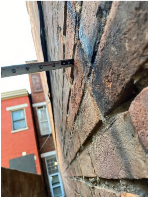
Photo 31 – Left Exterior, Localized Brick Joint Weathering
