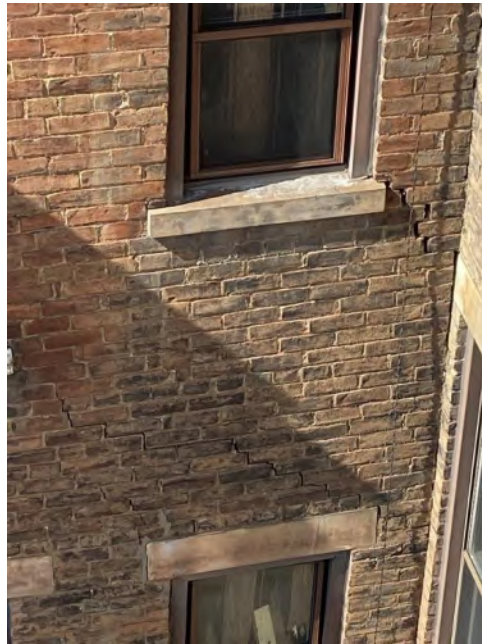
Photo 20 – Brick Settlement Cracking Above Covered Entryway, Rear Left Exterior
