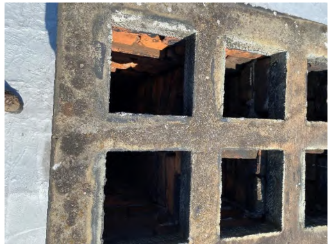
Photo 24 – Typical Open Flue
