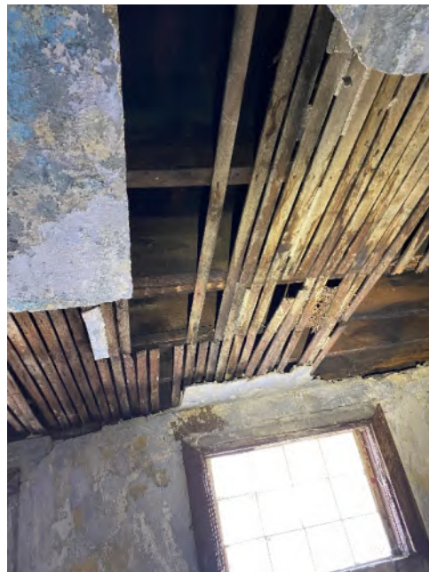
Photo 24 – Attic Framing, Some Previous Water Damage to Ceiling
