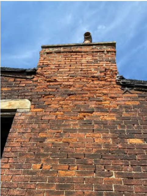
Photo 27 – Brick Spalling at Chimney
