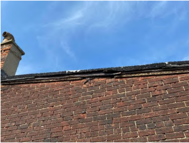
Photo 29 – Weathered Trim and Fascia, Left Exterior
