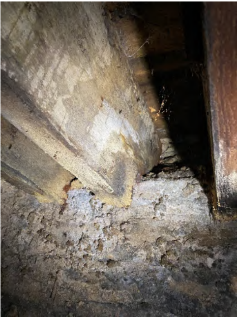
Photo 7 – Typical Joist Bearing and Moisture Damage, Left Foundation Wall
