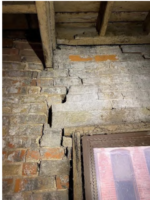
Photo 12 – Brick Movement at Rear Basement Window Due to Corner Settlement
