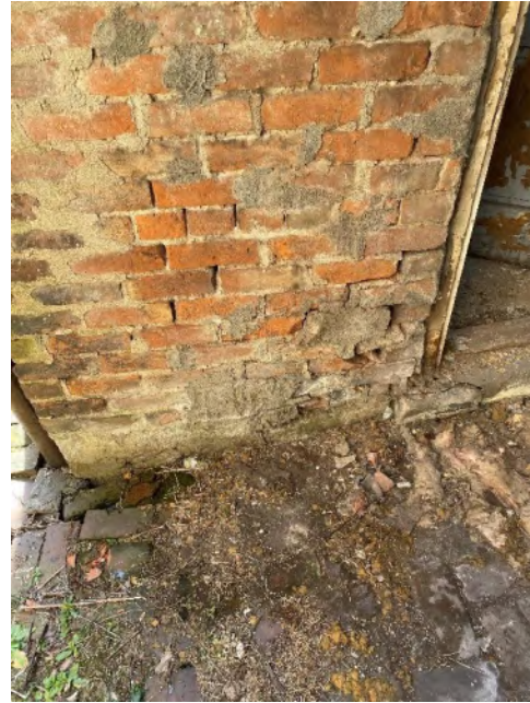
Photo 8 – Brick Joint Erosion and Weathering at Basement Corner
