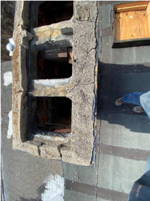
Photo 17 – Open Flue in Chimney
