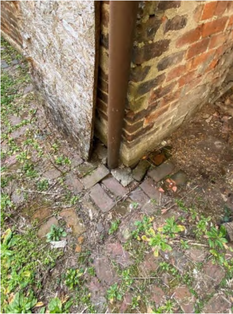
Photo 7 – Depressed and Eroded Soils at Settled Foundation Corner
