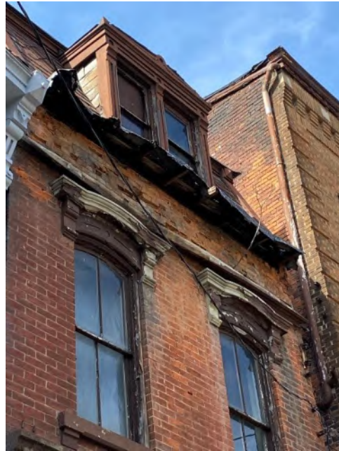
Photo 18 – Brick Spalling and Soffit Damage, Upper Front Wall
