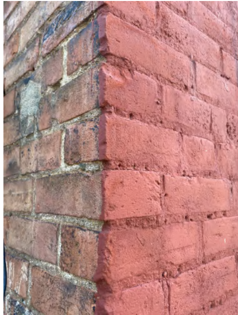
Photo 31 – Brick Condition, Front Face vs. Side Face
