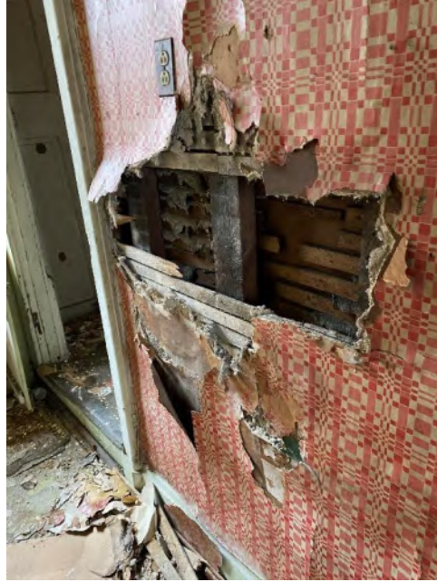
Photo 10 – Typical Plaster Damage, Interior Wall
