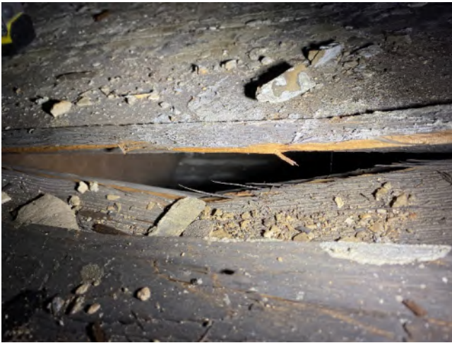
Photo 19 – Local Damage to Flooring
