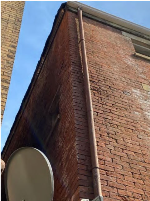
Photo 19 – Brick Joint Weathering, Back Left Corner at Downspout
