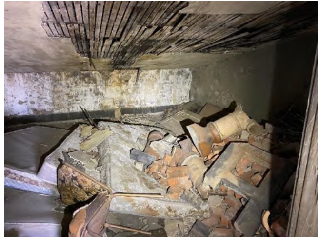
Photo 20 – Rubble and Brick Pile, Attic
