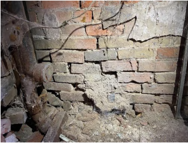
Photo 5 – Eroded Basement Wall Joints
