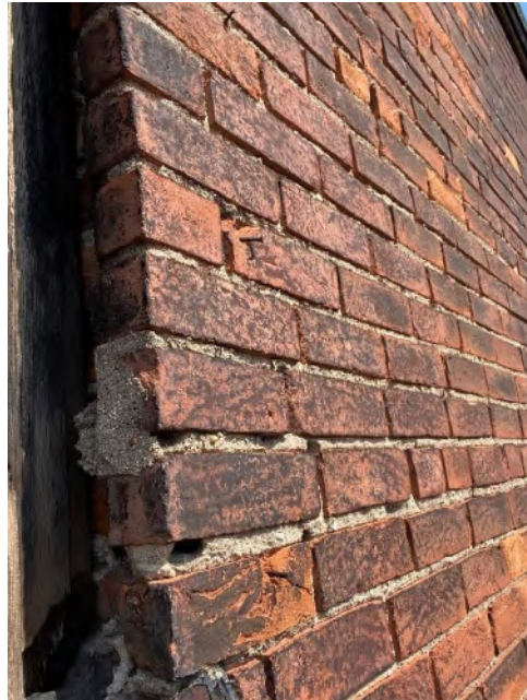
Photo 30 – Brick Joint Weathering at Window Opening
