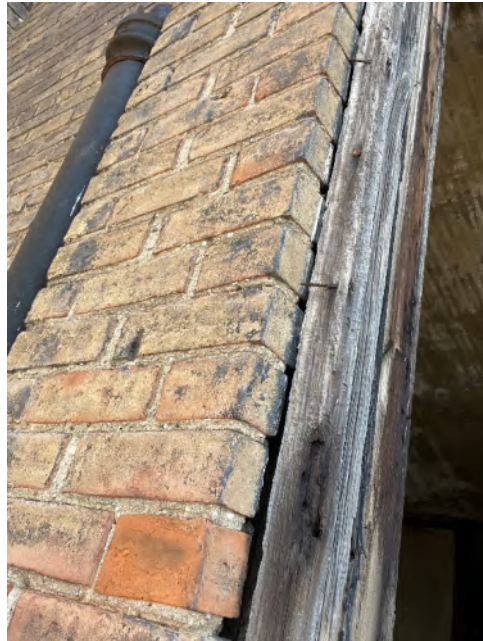
Photo 26 – Weathering at Missing Window, Attic Level
