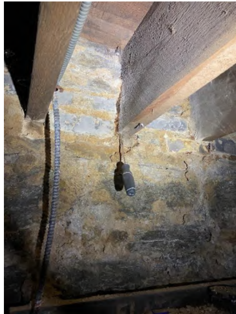
Photo 4 – Soft Rot at Bearing Ends of Left Floor Joists
