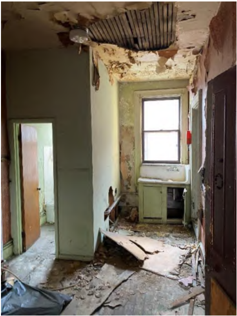
Photo 11 – General Second Floor Level and Ceiling Plaster Damage
