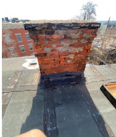
Photo 16 – Spalled Brick at Chimney
