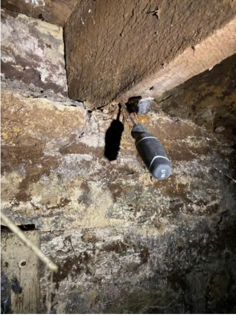
Photo 9 – Typical Soft Rot Damaged Joist Bearing End
