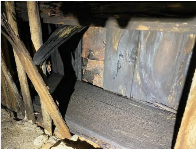
Photo 19 – Evidence of Previous Water Penetration, Front Left Demolished Chimney
