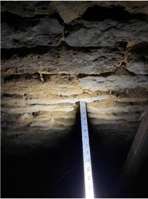
Photo 5 – Center Foundation Wall Joist Erosion Measurement
