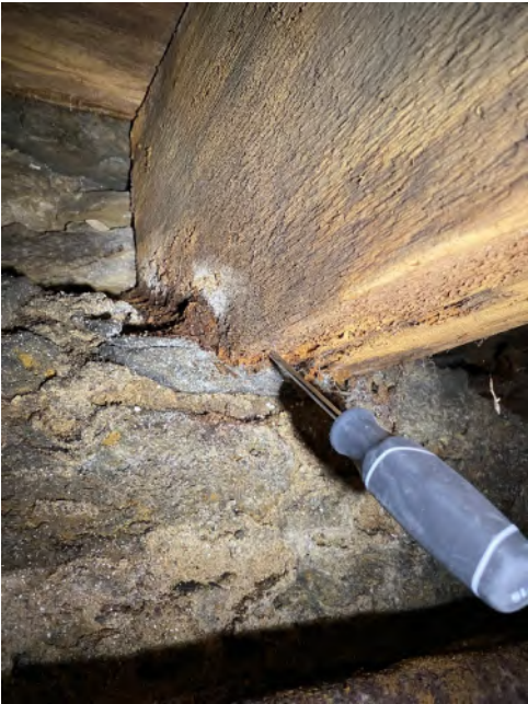
Photo 5 – Soft Rotted Joist Bearing End, Left Foundation Wall
