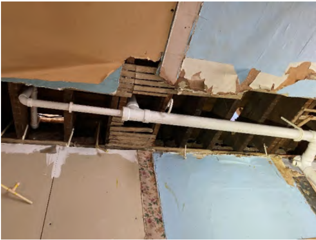
Photo 15 – Typical Plumbing, Missing Ceiling
