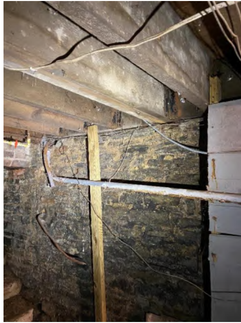
Photo 6 – Typical Header and Trimmer Framing, Left Foundation Wall
