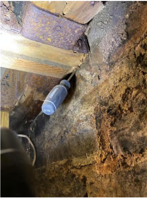
Photo 7 – Soft Rot Damaged Joist Ends, Left Foundation Wall
