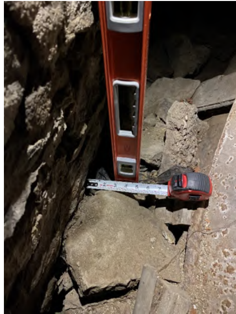
Photo 10 – Front Retaining Wall Bow Measurement
