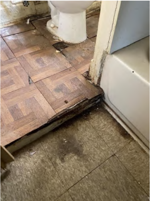
Photo 25 – Moisture Damage, First Level Bathroom
