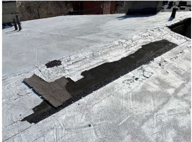
Photo 30 – Area of Roof Membrane and Shingle Damage
