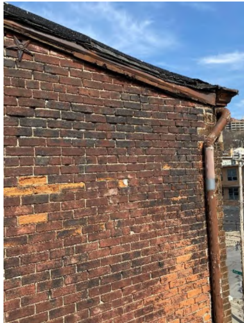
Photo 28 – Brick Joint Weathering, Upper Left Exterior
