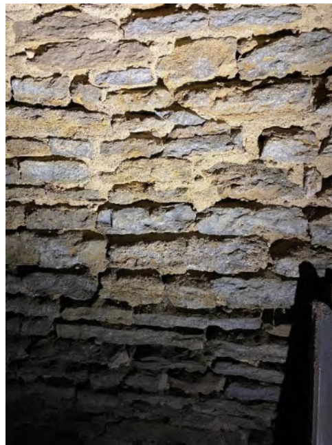
Photo 4 – Center Foundation Wall Joist Erosion
