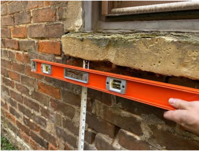
Photo 9 – Wall Slope Measurement Towards Settled Corner
