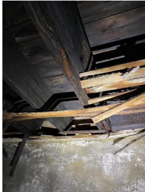
Photo 18 – Water Damaged Joist at Center Chimney
