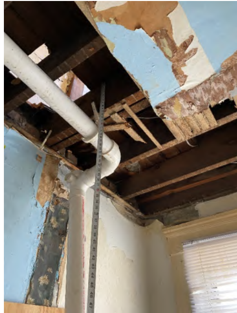
Photo 14 – Typical Plumbing, Missing Ceiling
