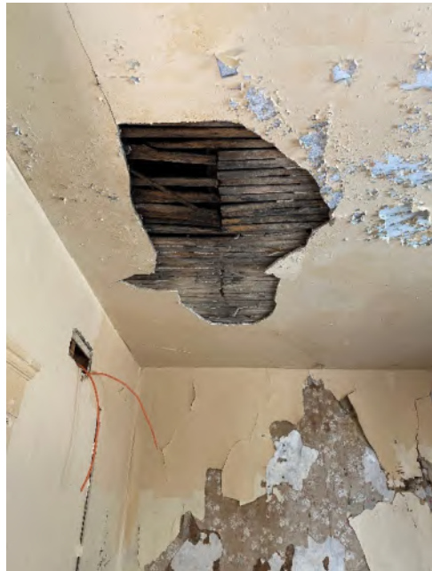
Photo 20 – Typical Plaster Damage, Likely Plumbing Related
