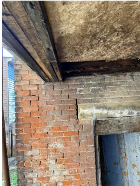
Photo 10 – Brick Movement at Rear Basement Door Due to Corner Settlement
