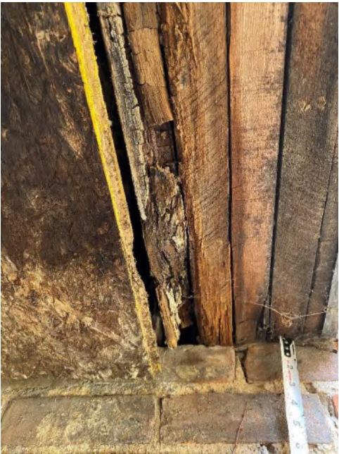
Photo 15 – Damaged Built-Up Floor Beam at Covered Entryway
