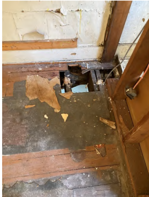
Photo 18 – Floor Penetration Below Plumbing Area
