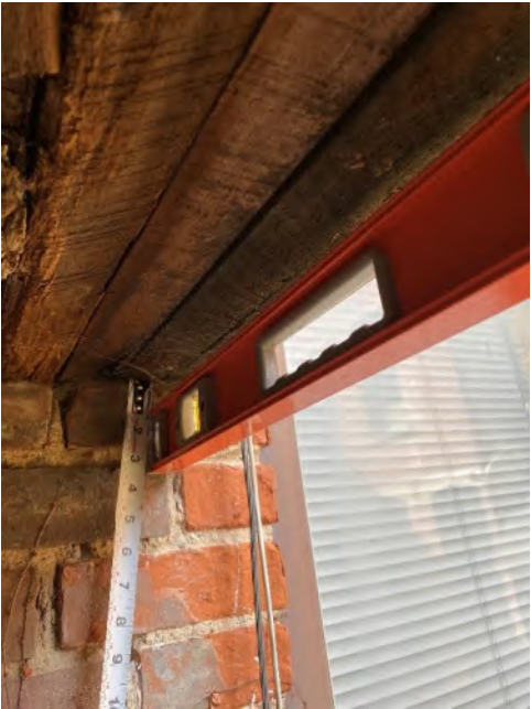
Photo 13 – Floor Beam Tilted Towards Settled Foundation Corner
