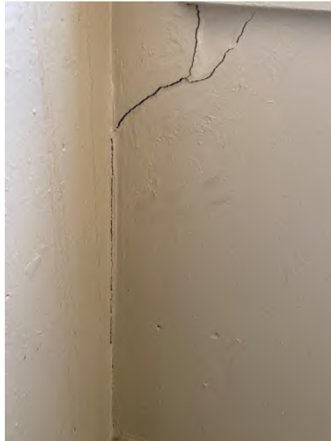
Photo 30 – Plaster Crack from Foundation Settlement
