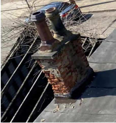
Photo 33 – Rear Right Spalling and Deteriorating Chimneys
