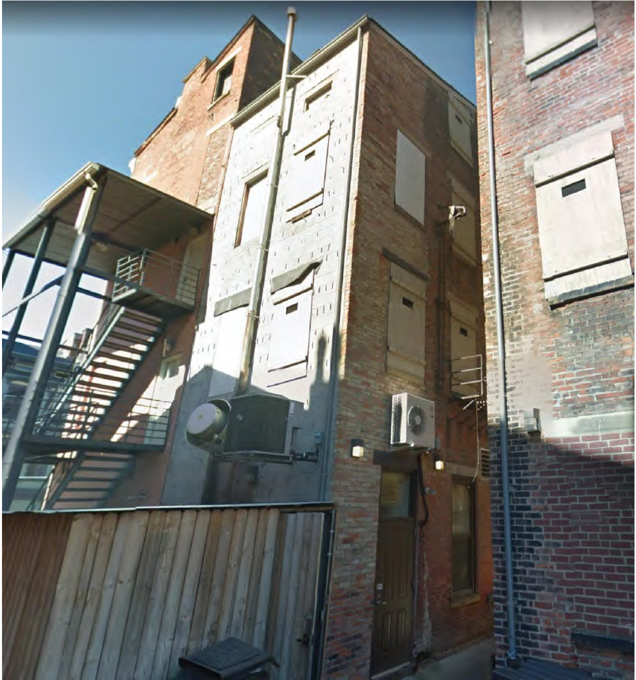
Figure 3: The rear of 133 W Elder Street with exposed CMU and brick ties for the promised brick
