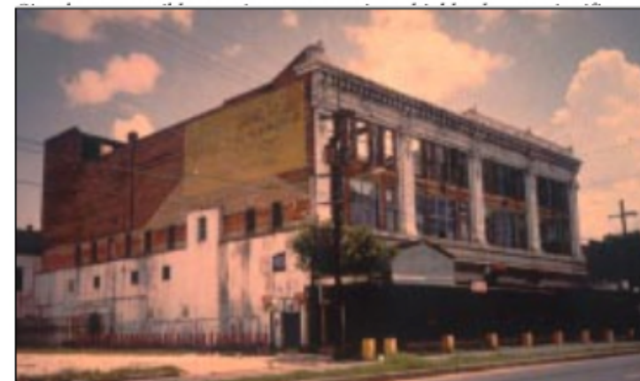
The side elevation of a 1914 department store featured several non-historic openings which had been added over the years.
