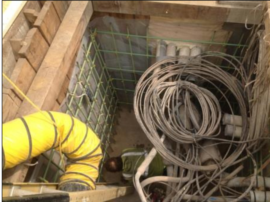
Cincinnati Bell Telephone vault on 12th St. at Race St.
