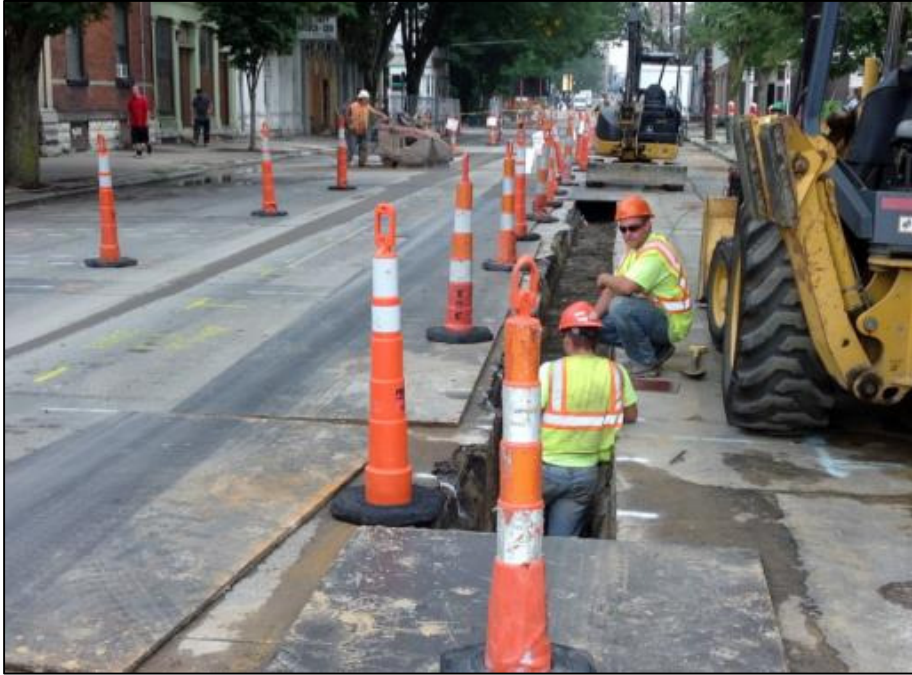
Duke Energy gas work on Elm St. between 14 th and Liberty St.
