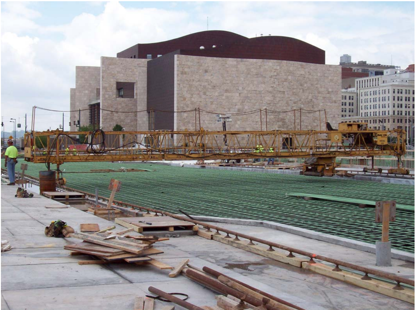
A Bidwell machine will be used to place and finish the concrete for The Banks' newest street, Freedom Way East, saving both time and money.
