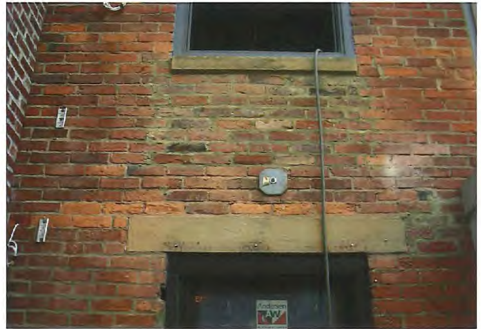
POOR EXISTING PATCH JOB EAST ELEV @ ALLEY
