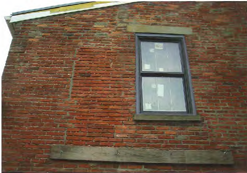
EAST ELEVATION - MISMATCHED BRICK FROM DIFFERENT ERAS
