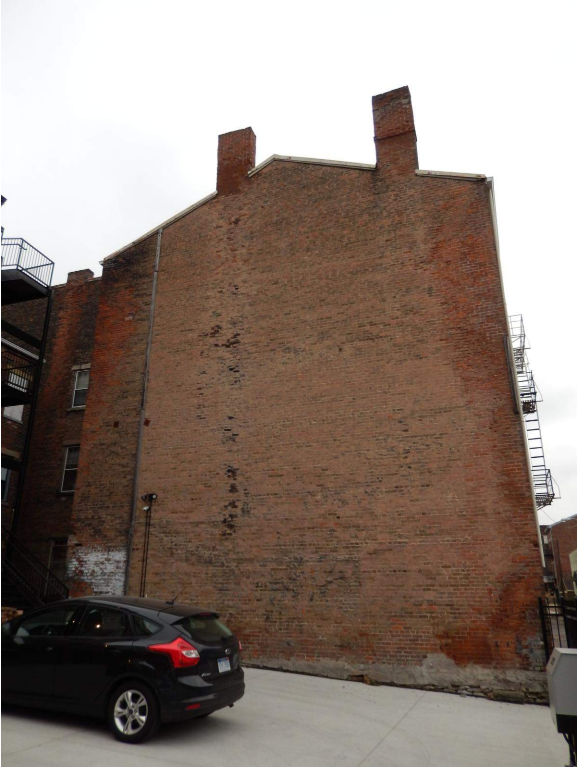
Rear Building - Elevation Facing Neighboring Parking Lot (North Elevation of Rear Building)
