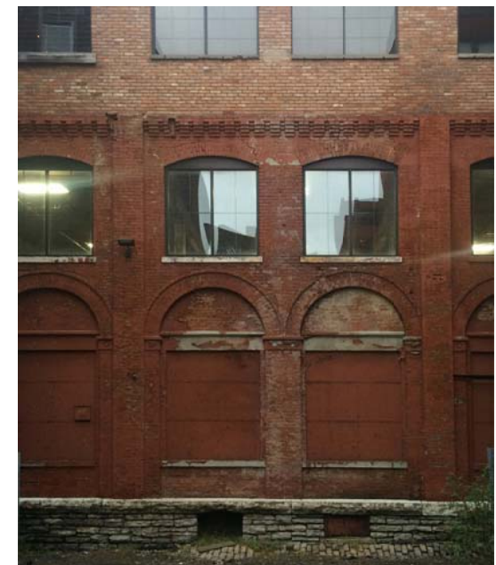
04 VIEW OF EXISTING ETON PLACE FACADE - EXISTING METAL WINDOWS AT GROUND FLOOR REPAIRED AS NECESSARY
