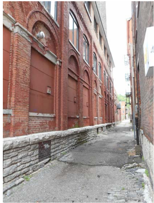
03 VIEW DOWN ETON PLACE - ORIGINAL WOOD WINDOWS AT GROUND FLOOR REPAIRED AS NECESSARY
