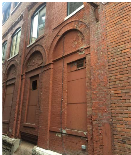
05 VIEW OF EXISTING ETON PLACE FACADE - INFILL EXISTING OPENING AT GROUND FLOOR, HOLD MASONRY BACK 1" FROM FACE
