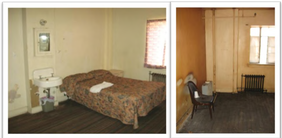
Current Unit Conditions
